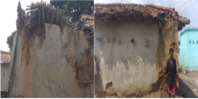
Figure. 24. a) & b) Menace of uncontrolled blasting in Urub Dalit basti of Bhuiyans
